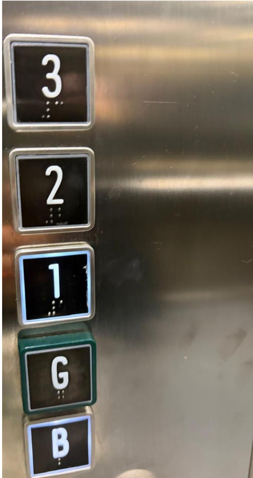
Braille-labelled elevator control panel
