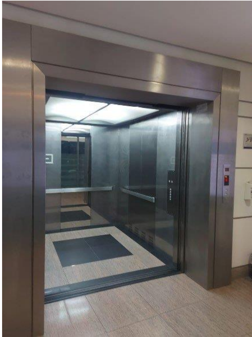
Elevator suitable for use by PwD
