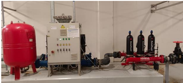
Irrigation Pump Station
